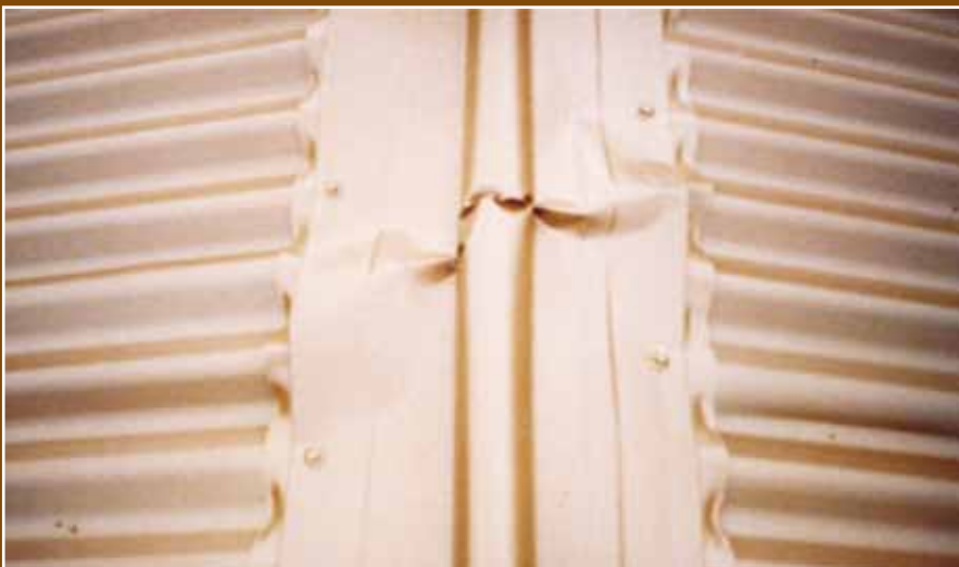
Buckled roof capping
